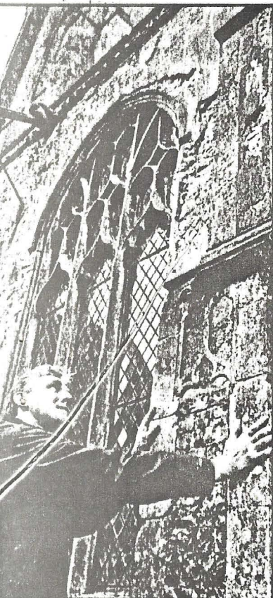
The chairman of the Friends of St Agnes' Church, Cawston, John Farrow, examines the decaying masonry of the south aisle.
